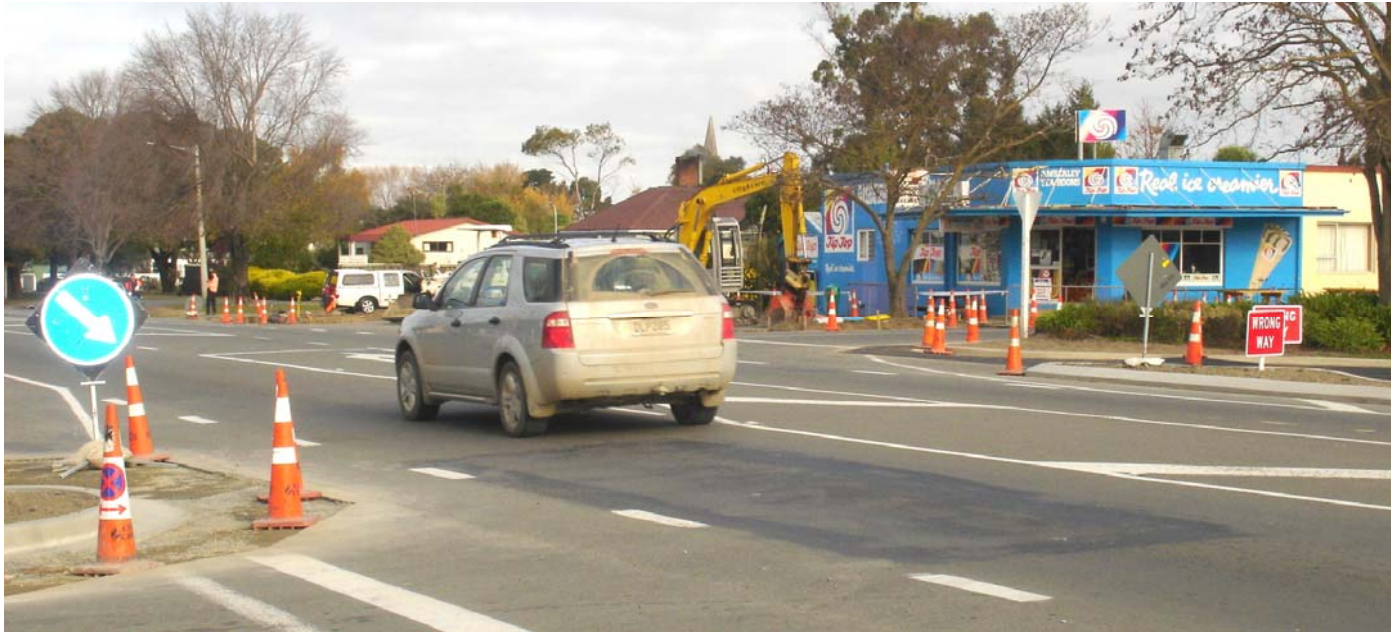
While work is progressing rapidly it is still a 'work in progress'
