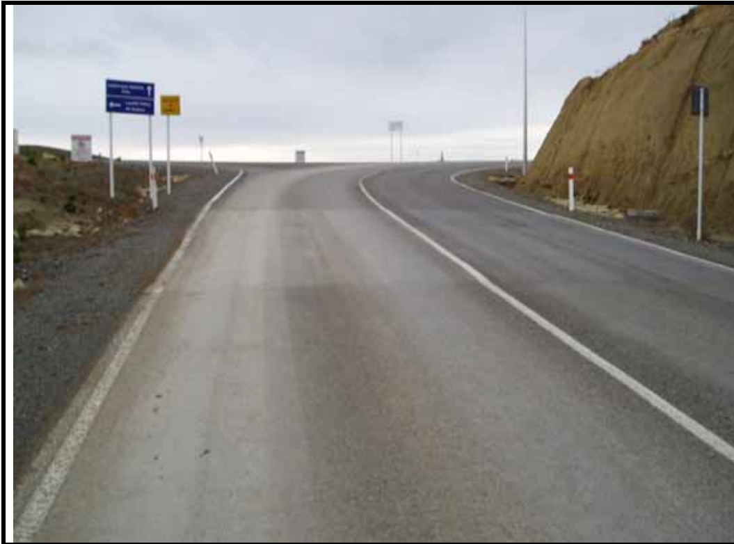
Description: Peek counter / classifier on LAR. The piezometer tubes are in the downhill(outward) lane.
