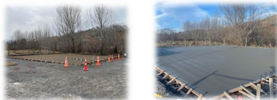
Green waste area at Hanmer Springs transfer station excavated, compacted with the steel installed pre-pour and post-pour.
