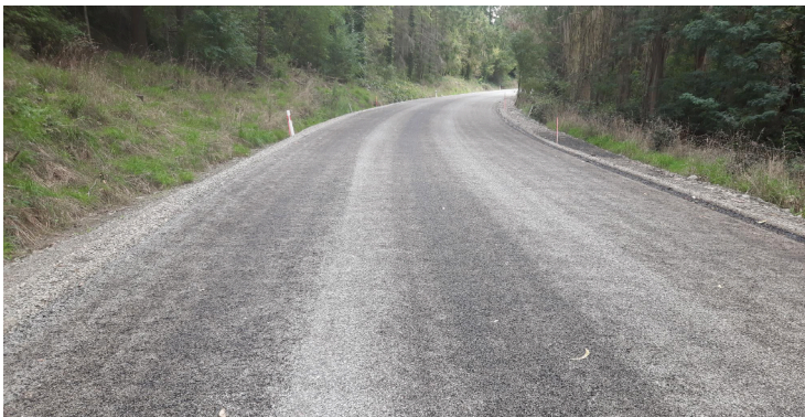
Improvement works to strengthen the road pavement and improve drainage on Factory Road, Cheviot, are near completion, with works planned to be completed in early April.
