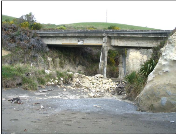
Figure 8.2: Rail bridge over Claverley Road 500 m north of Claverley settlement (photo DTec, 2004)
