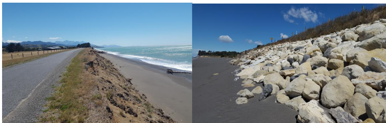
Figure 7.2: Conway Flat Road: (a) Road close to alluvial cliff edge; (b) Armour rock protection on cliff face and toe.
