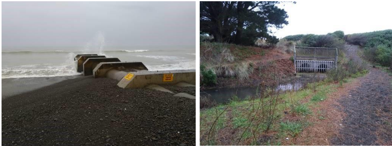
Figure 3.2: Leithfield Beach drainage outfall pipe in centre of the settlement; (a) the Ocean outfall; (b) pipe inlet at the back of the beach ridge.
