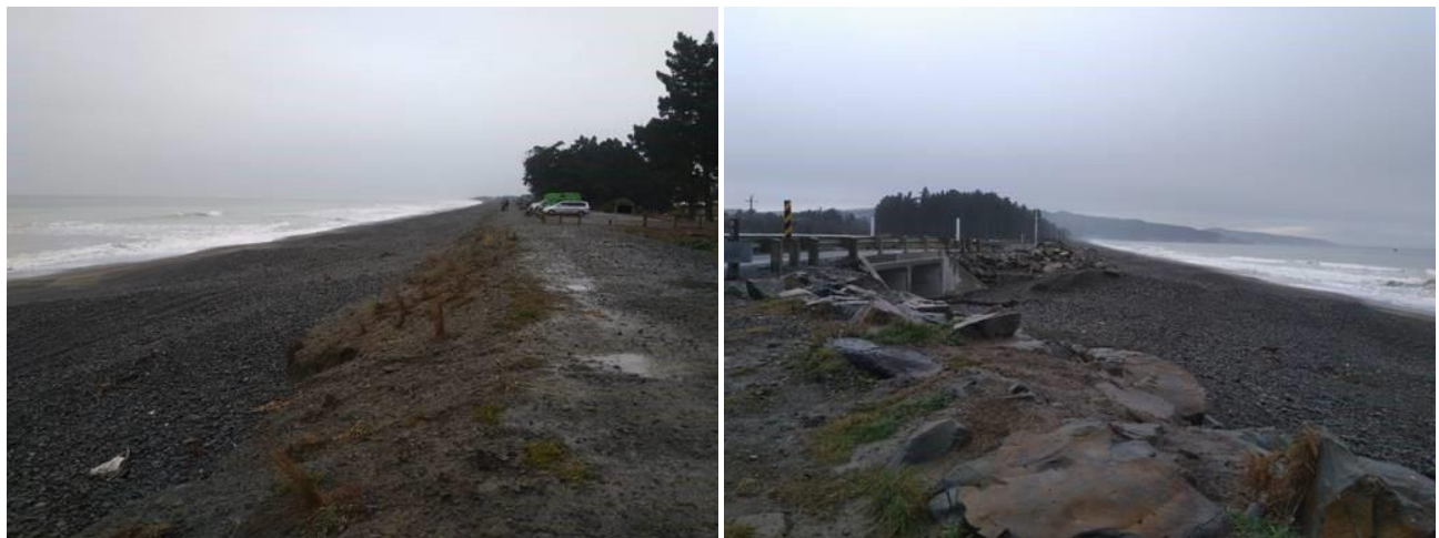
Figure 4.2: (a) 1km Bund along the storm ridge at Amberley Beach (photo July 2019), (b) northern lagoon inlet under the bridge at Golf Links Road, an identified piece of critical infrastructure.
