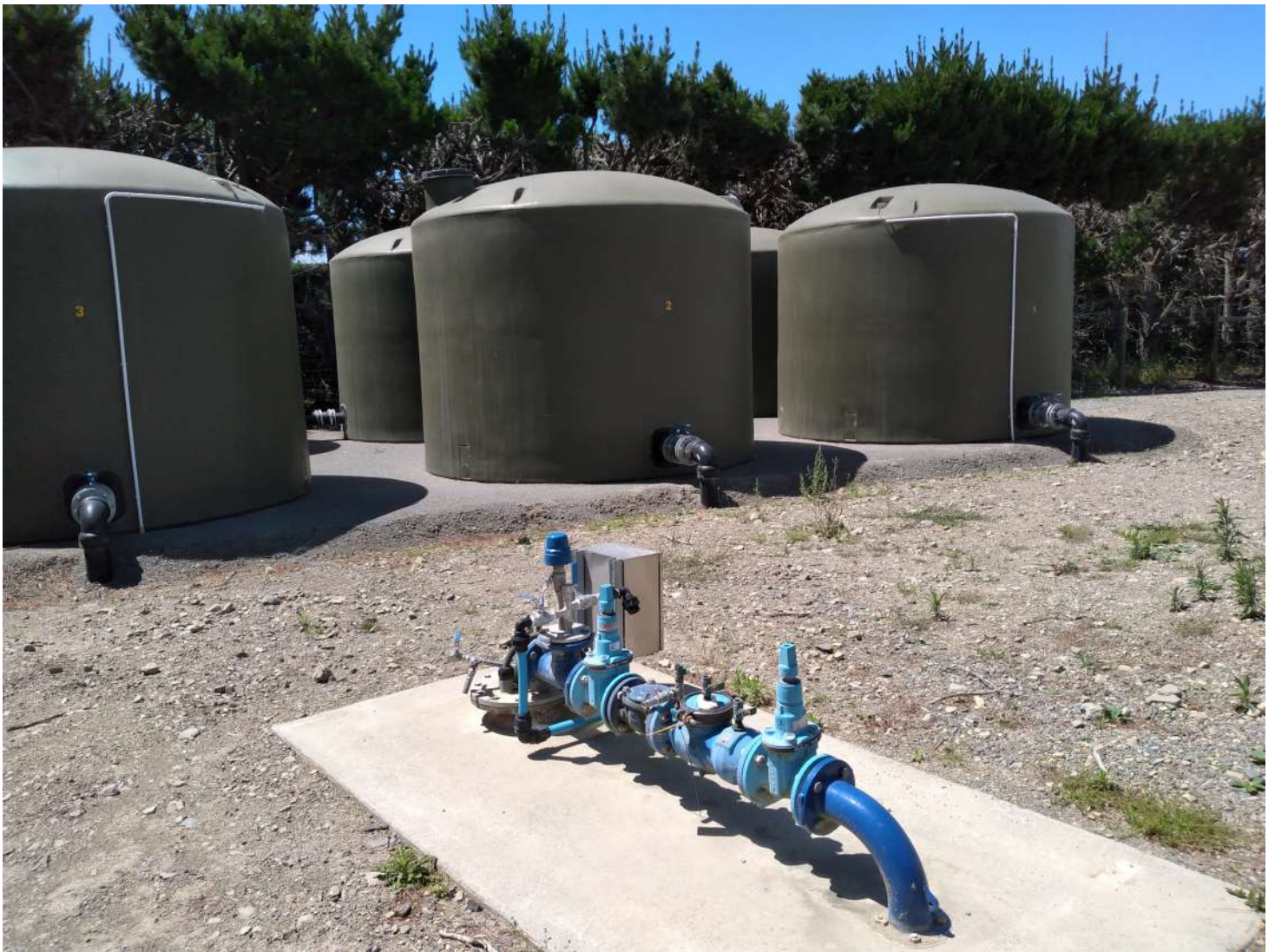
Water tanks at the Racecourse Road water treatment plant, Amberley.
