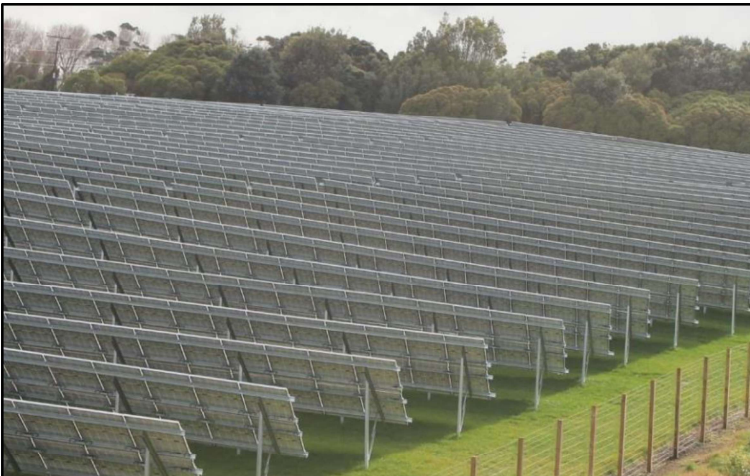
Figure 10: A similar PV module arrangement at the Kapuni Solar Farm, Taranaki. The photo shows that grass coverage over the ground is practically unchanged because of the PV modules.
