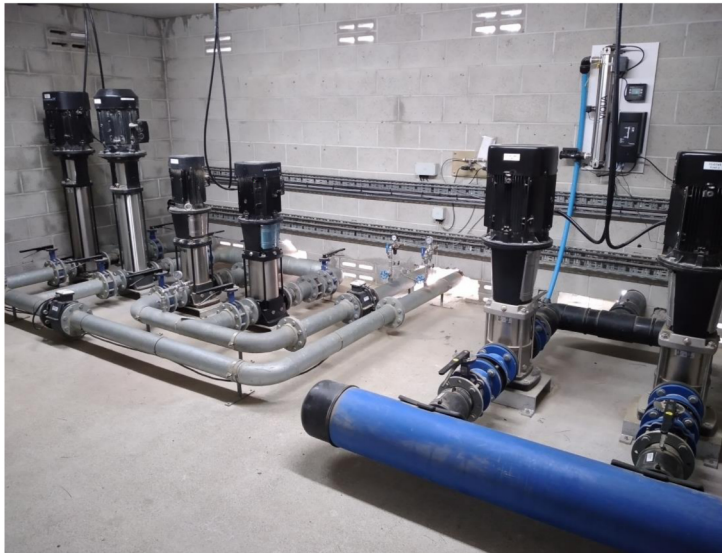
Race Course Road Water Treatment Plant, Amberley
