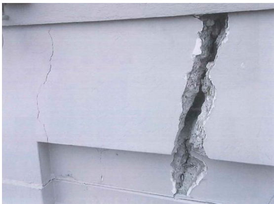
Photo 5 – Crack identified to external of West elevation above west blockwork extension.
