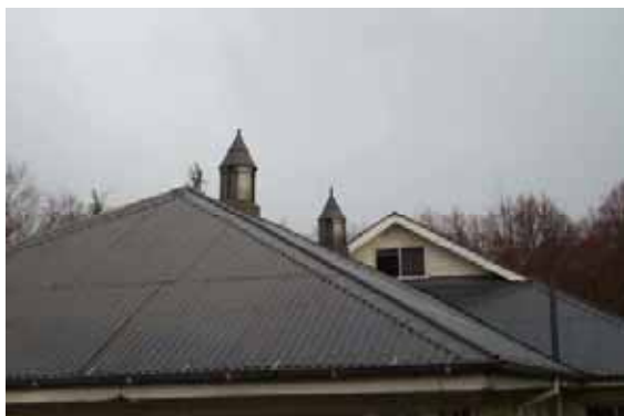
Gymnasium Building, Roof of eastern end in foreground, with ventilators, and roof of block with cubicles shown offset at rear.
