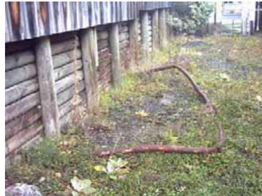
Main Pool pipe?
