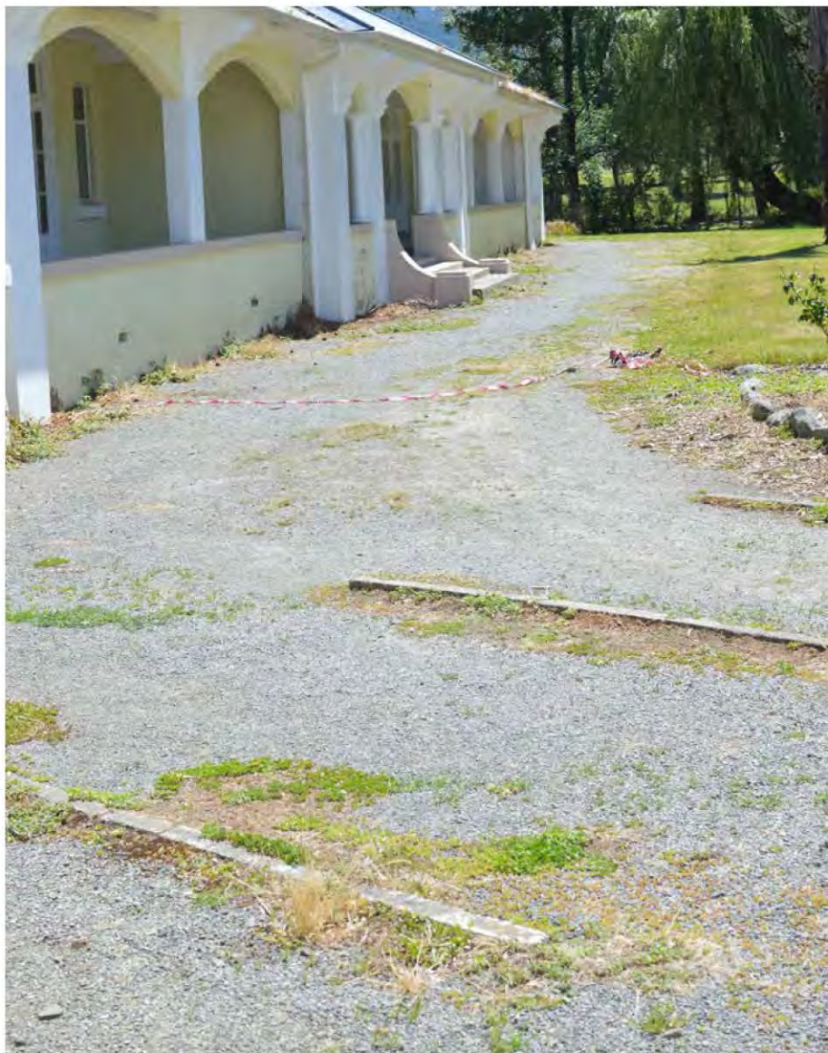
Photograph 16. Uneven surface along east side of Chisholm Ward
