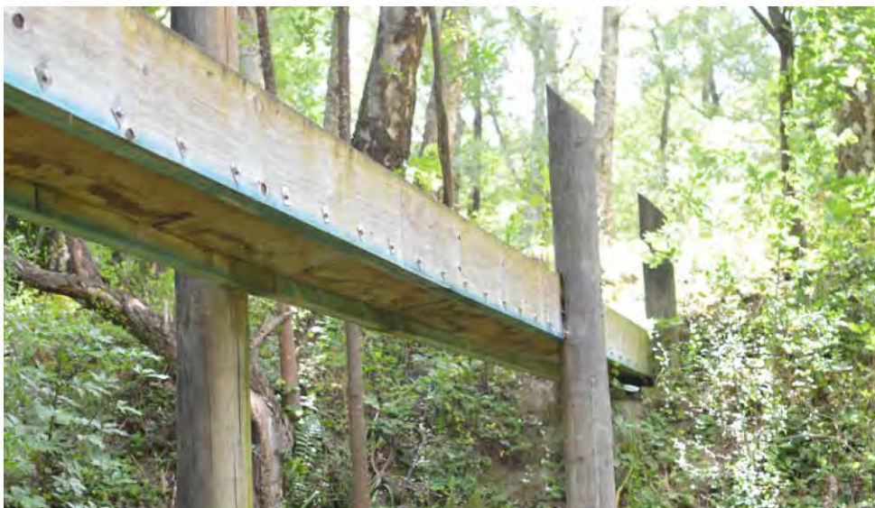
Photograph 5. Overhead services cross Hospital Stream boardwalk
