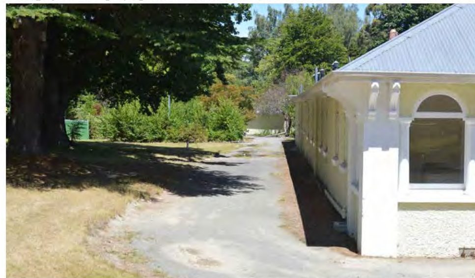
Photograph 19. Eastern side of Chisholm Ward with puddles, weeds and hazard tape across path
