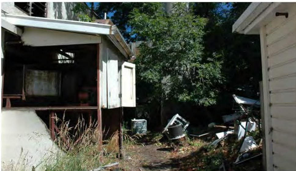
Photograph 39. Derelict buildings and rubbish adjacent to the Blacksmiths Cottage with access to Public Cottage
