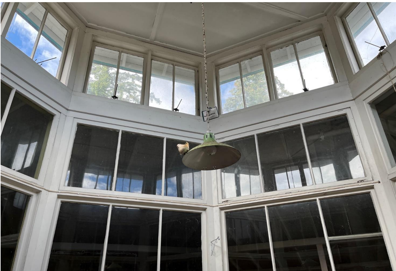
Lantern within nurses station in eastern ward
