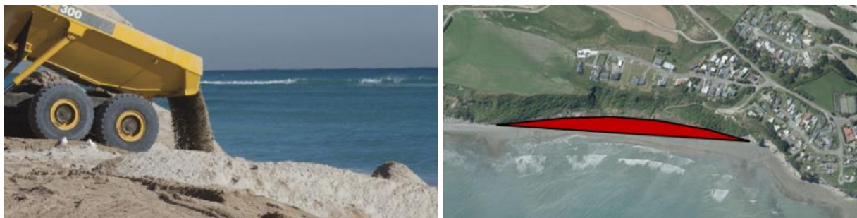
Figure 4.7: (left) Sand renourishment; (right) approximate area of Sandy Bay where sand would be placed.
