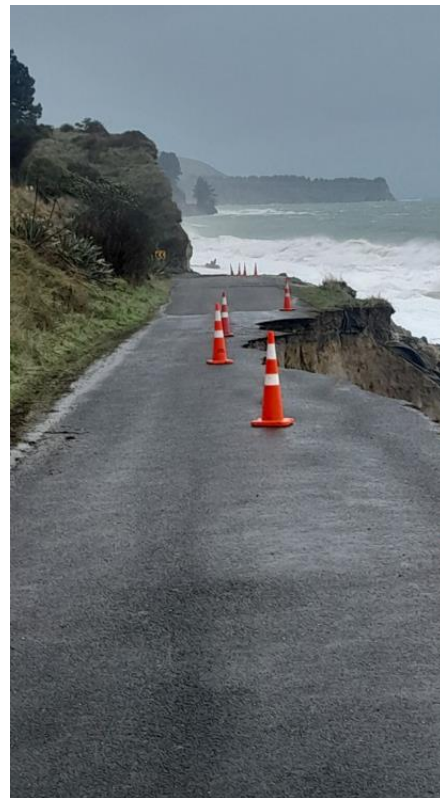
Damage at Claverley Road 2023
