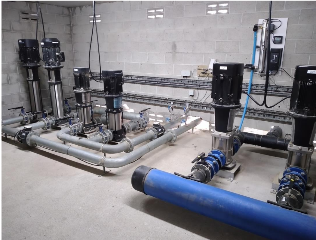
Race Course Road Water Treatment Plant, Amberley
