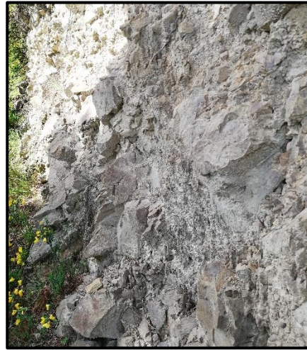
Photo 2: Observed cut slope above walking track, indicating near surface Weathered in situ Greywacke Sandstone
