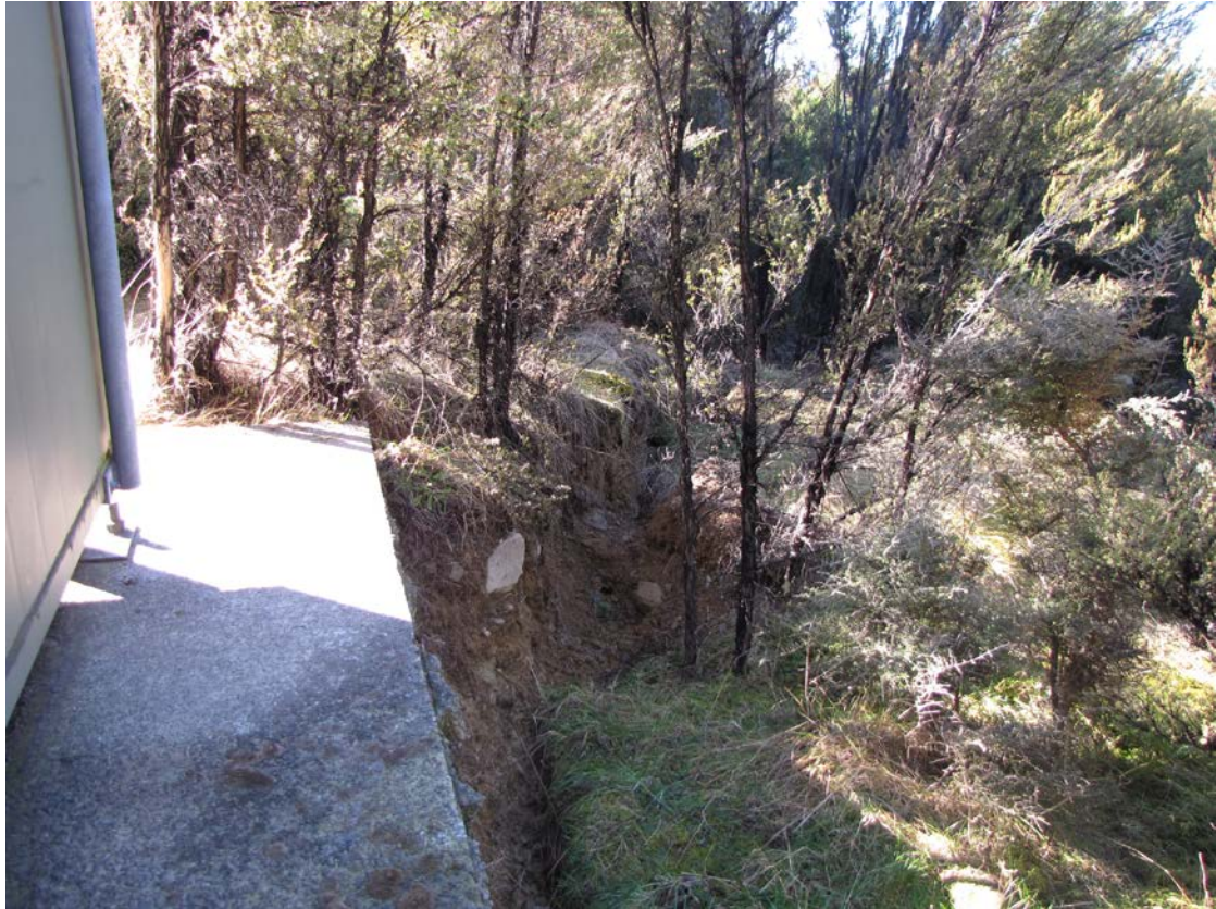
Figure A1.7 Down-slope ground failure related to slope instability at the Spark repeater, Tinline Terrace. The scarp in the centre is c. 0.6 m high.
