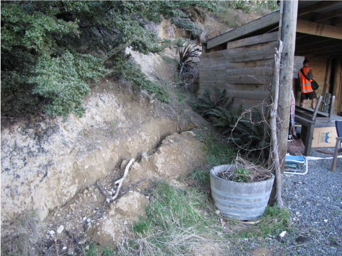
Figure A1.11 Arcuate slope cracking and extension at the edge of a steep cut slope at property on Terako Terrace.
