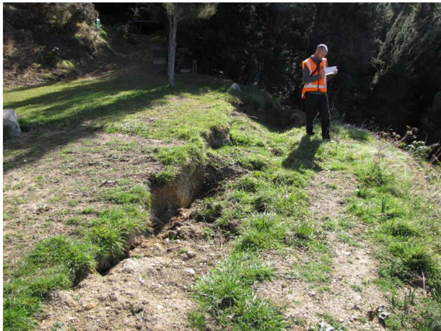
Figure A1.14 Ground cracking and extension causing subsidence in a yard at a property on Lulus Lane, adjacent to a steep cut bank edge.
