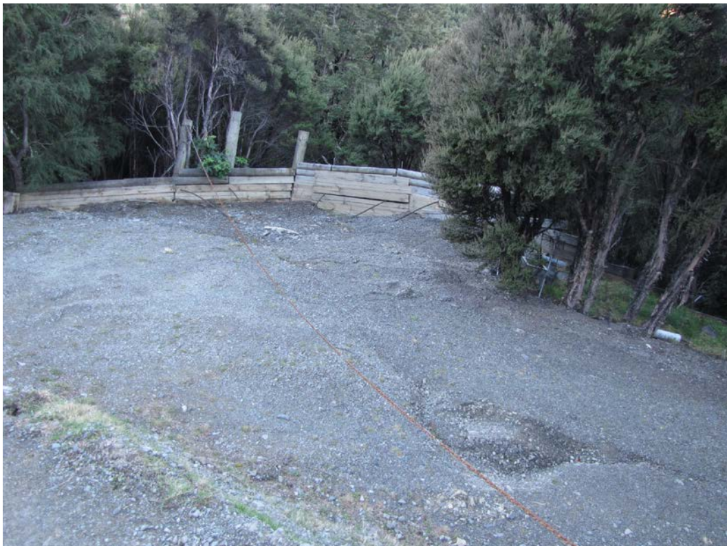
Figure A1.12 Arcuate cracking and extension in fill forming an off-street parking pad supported by a retaining wall adjacent to a property on Cloudy Range Road.
