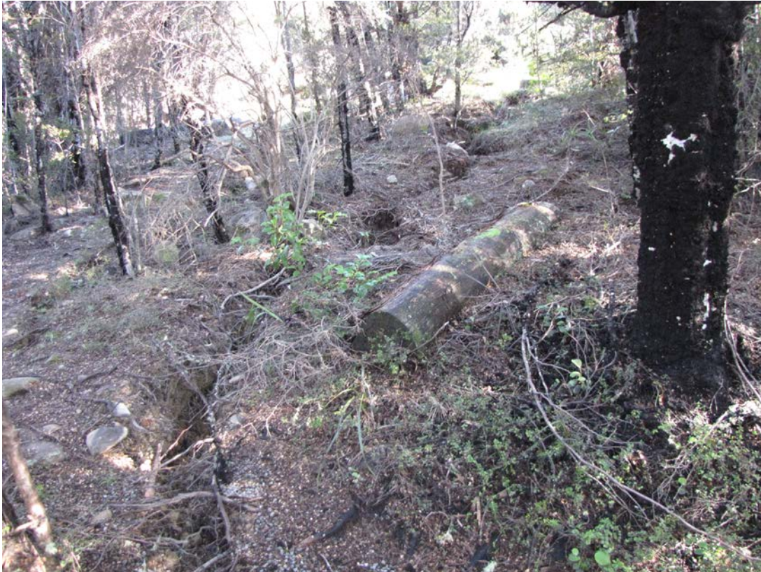
Figure A1.5 Arcuate ground cracking related to slope extension within scrub above 'unnamed' stream.
