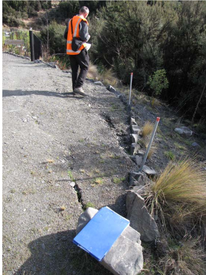
Figure A1.13 Cracking and extension in fill at the edge of a driveway approach above a steep slope adjacent to a property on Mt Lyford Drive.
