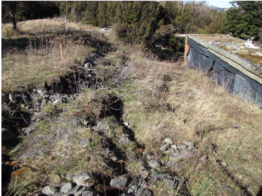
Figure A1.8 Typical slope extension and ground failure above a cut slope where structure has been erected. Site is above the SW edge of 'unnamed' stream.
