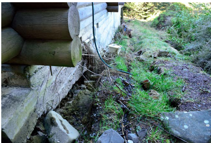
Figure A1.2 Typical ground extension observed at the downhill-facing edge of a house at Mt Lyford Village.
