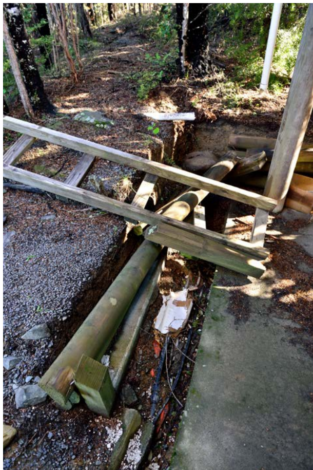
Figure A1.1 Typical foundation settling adjacent to a split-level log house at Mt Lyford Village. Note the subsidence of the ground and ground cracking extending away from the house (concrete pad).
