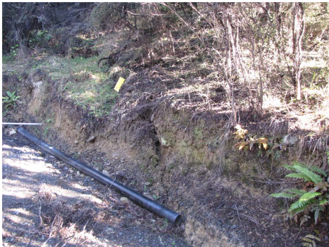
Figure A1.6 Ground cracking and downslope failure (projecting to back of photo beyond yellow notebook) of c. 20 cm, exposed in a car parking bay cutting.
