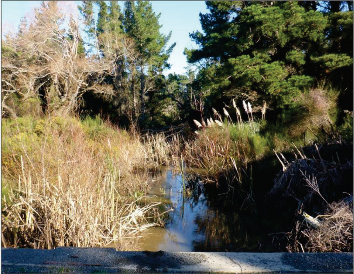
Figure 2-10: Eastern Drain looking downstream from Amberley Beach Road at the twin culverts
