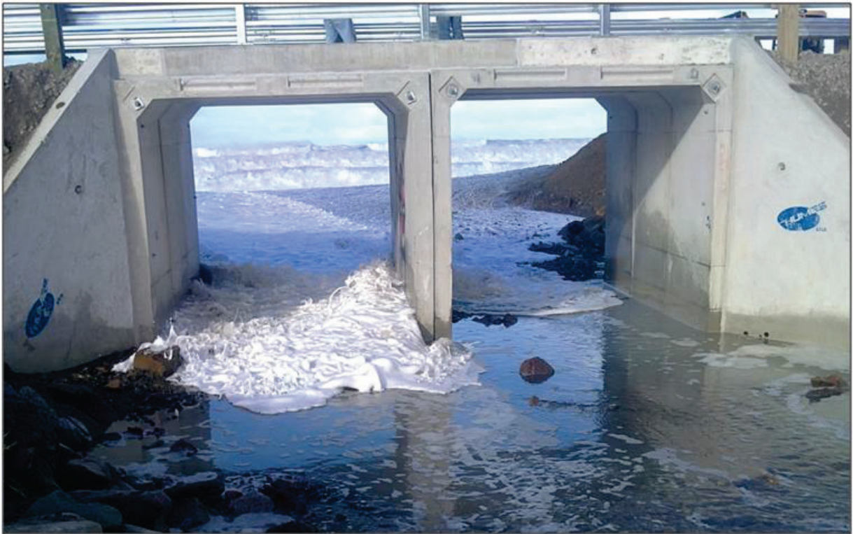
Figure 2-7: The new Amberley Beach (Northern) Lagoon outlet structure showing sea water passing back into the drained lagoon (Photo: Ross Harper)
