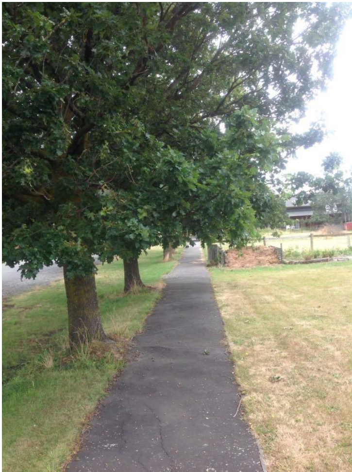
Street trees overhanging footpath and roots causing the footpath to lift (Rotherham)
